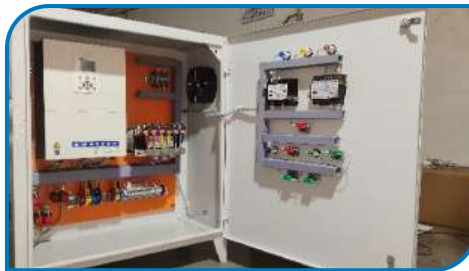
SOLAR VFD PANEL
