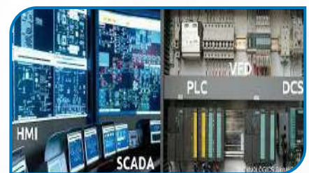
SCADA/DCS/HMI DEVELOPING LABELLING
